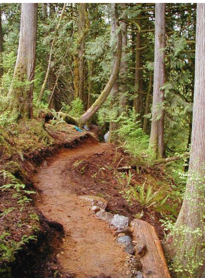
Newly completed section along the Lime Kiln Trail. Photo courtesy Bob Chesterman. (May 2003)
