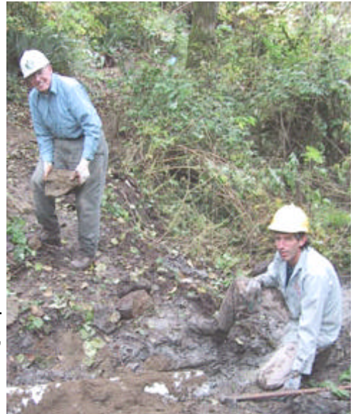
Trail veterans Duane Acheson and Jim Oosterhof construct rock headwall for culvert installation near
